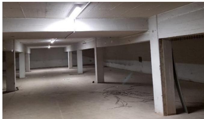
Fig. 1: Cellar with bearers and columns which is to be transformed into a hot water storage [Source: Own illustration]
